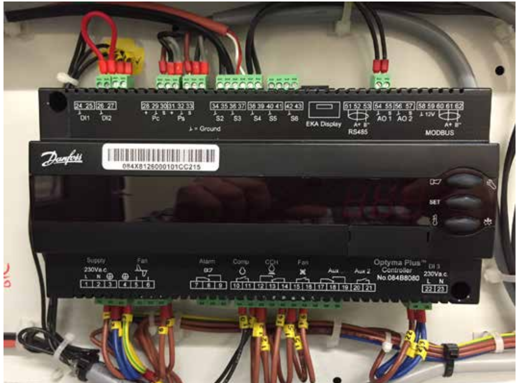
Picture1. Normal wiring
